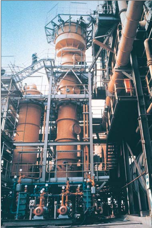
Fig. 18: Chlorine filtration plant
