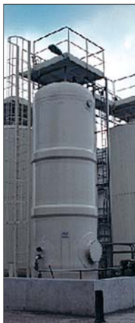
Fig. 37: Storage tanks for chemicals
